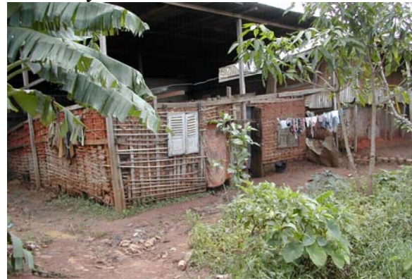
... Poor quality of houses
